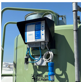
Mandatory leak detection system
