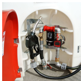
Fuel transfer unit
