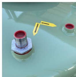
Detail of suction and return lines
