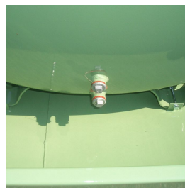
1" drainage point for routine maintenance and cleaning
